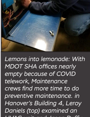
Lemons into lemonade: With MDOT SHA offices nearly empty because of COVID telework, Maintenance crews find more time to do preventive maintenance. In Hanover’s Building 4, Leroy Daniels (top) examined an HVAC unit and Jason Duffy repaired a boiler.
